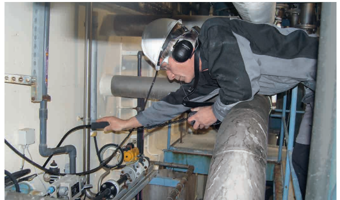
Leakage detection in the plant in Koog aan de Zaan. The detected leaks represent about 8% of total compressed air costs.
